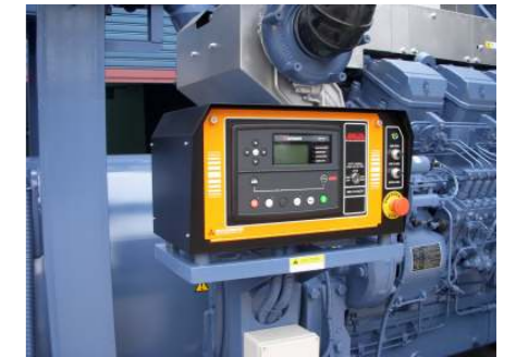
Mitsubishi Vietnam Ltd Generator Control Panels 1000 per year
