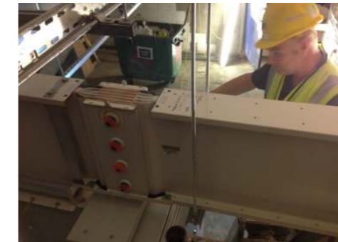
Silverline Constructions 4000 Amp Canalis Busbar 2013
